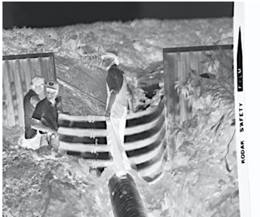
Figure 18. Photographic negative depicting the construction of a terrace in Benton Co., Indiana, Benton County SWCD
